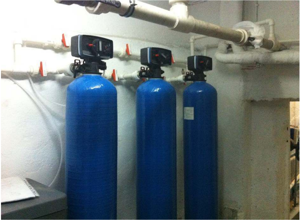
HAYAT APARTMENT — ANKARA/TURKEY — Drinking Water Treatment Plant, 10 m 3 /Day (2014)
