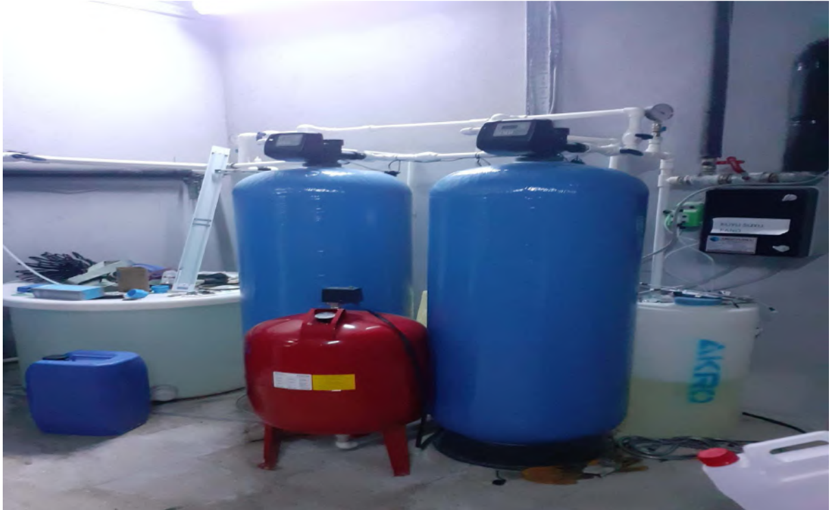
TITANIT CONSTRUCTION — KHURAI F-15 PROJECT/S. ARABIA — Water Treatment Plant, 240 m 3 /Day (2019)
