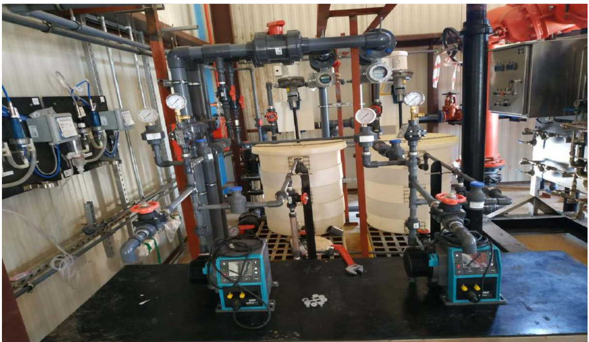
77 CONSTRUCTION — DJIBOUTI CAMP LEMONIER CHEMICAL DOSING — REPUBLIC OF DJIBOUTI — Chemical (Chlorine) Feed System and Carbonic Acid Feed System, 550 m 3 /Day (2019)
